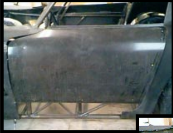
Shown above: Door skin is trimmed to fit the door opening and temporarily mounted using pop rivets.
